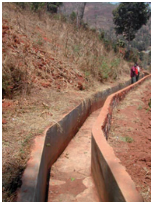
Kinko (Tanzania): Canal exposed to erosion and not covered
