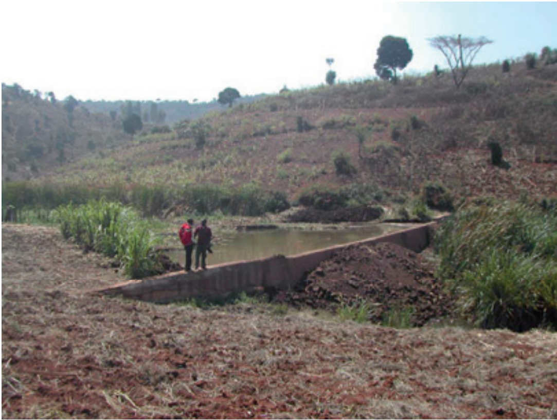
Kinko (Tanzania): Heavy silt load but no proper curing facility
