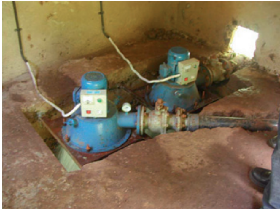
Kirinyaga (Kenya): Two chinese pico-turbines in parallel
